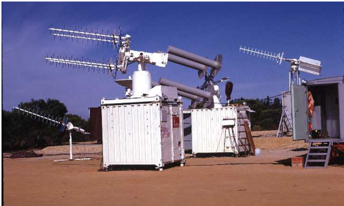
Figure 19: Telemetry reception complex.
